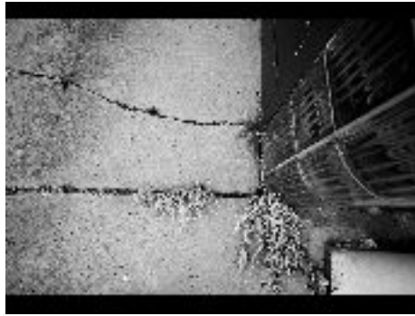
Cracks and Weeds
