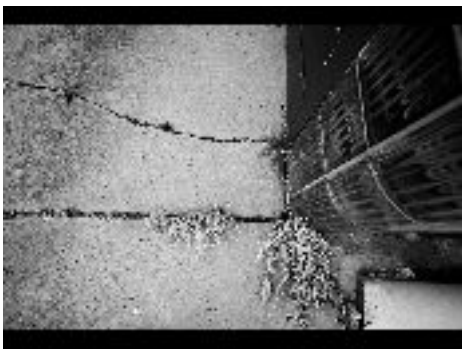
Cracks and Weeds
